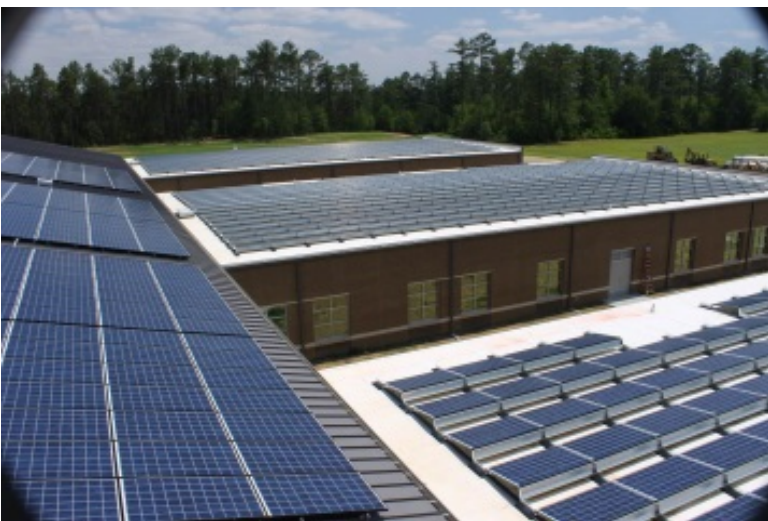
2,358 solar panels cover the entire roof of Sandy Grove Middle, producing enough energy to power more than 68
